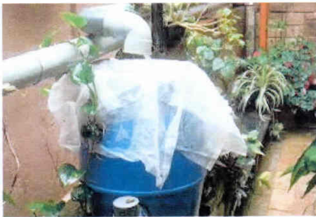
Water Storing In Tank
