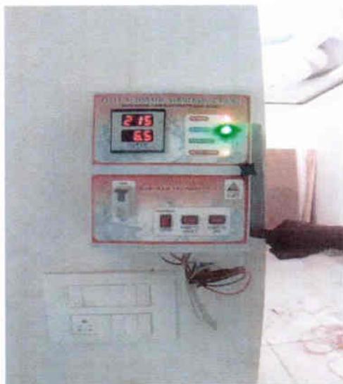
Automatic Pump Controller
