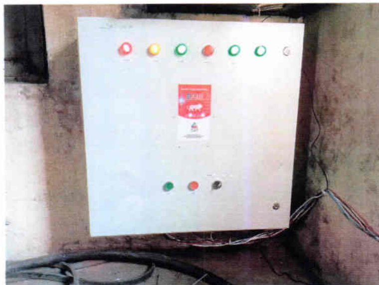
Scada Based Water Flow Control Panel
