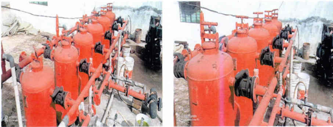
Filters and vanchury for centralized water Distribution
